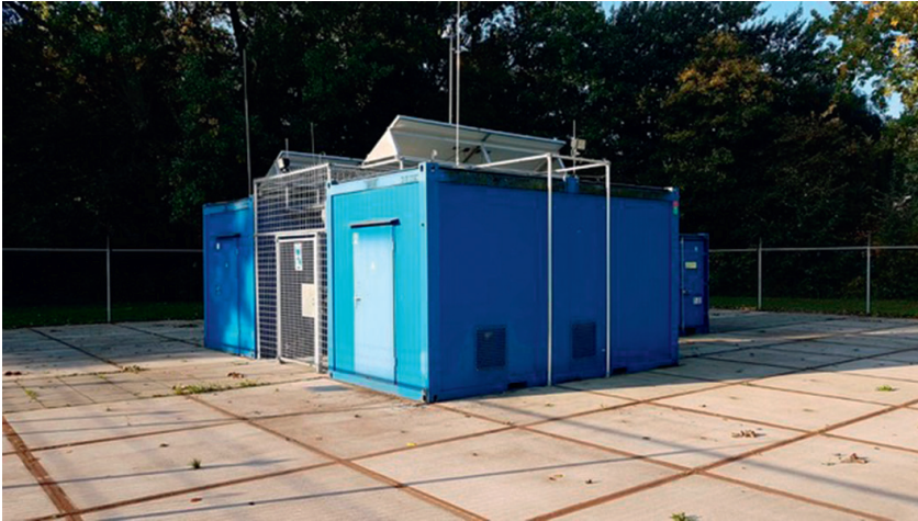
Figure 2. The hydrogen production unit at Rozenburg
